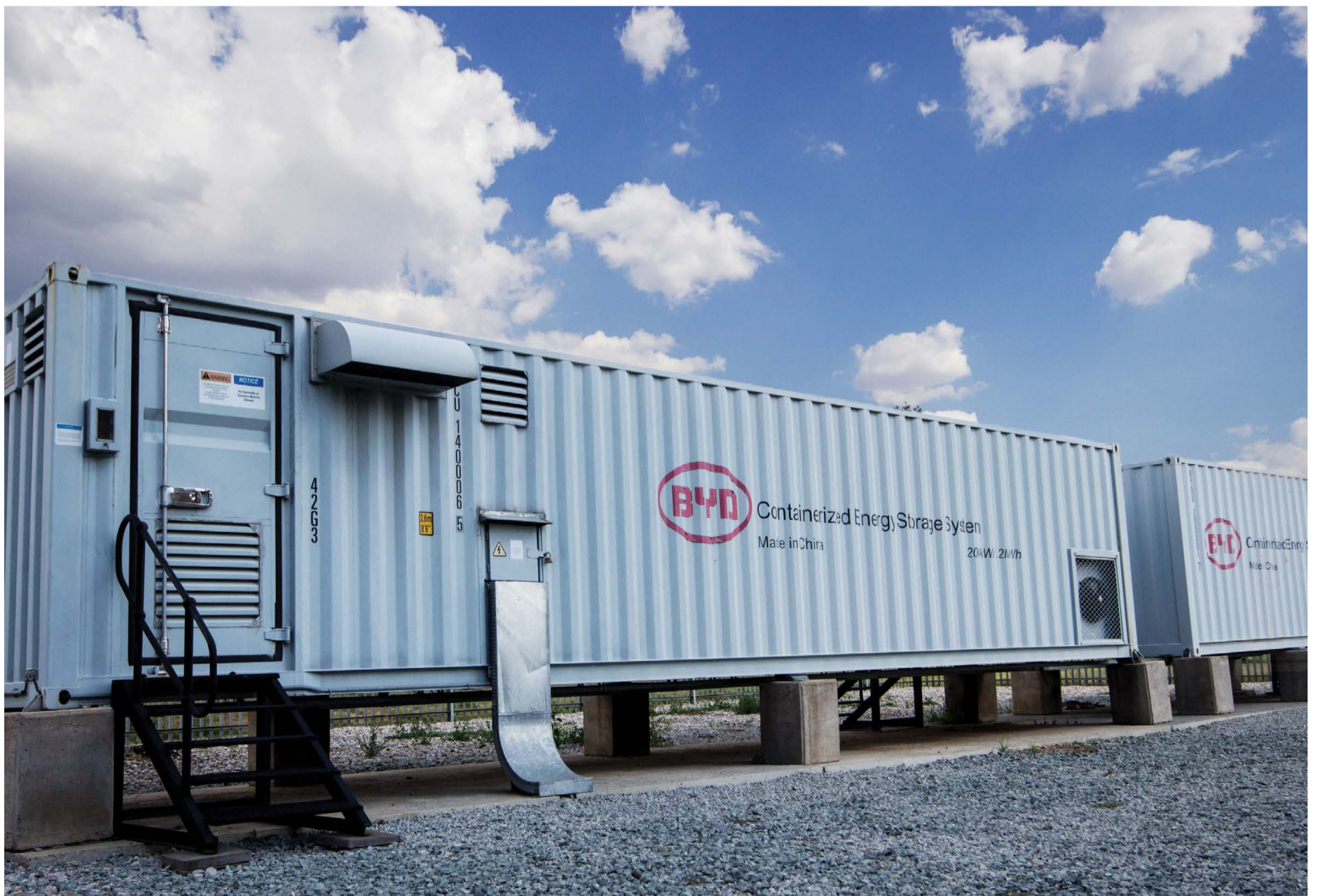
A container housing battery banks
